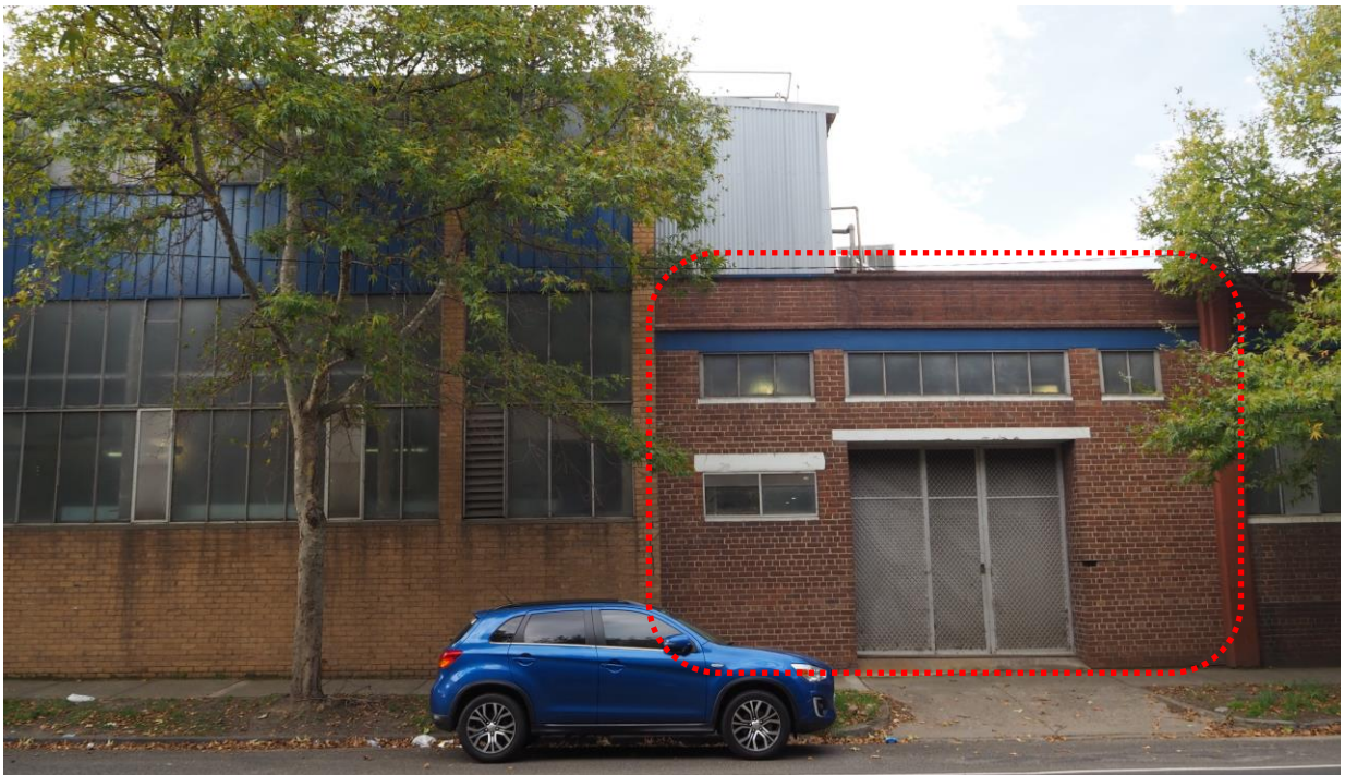
Addition to single-storey section of Glassmaking Plant (dashed) at the junction with the adjoining Postwar Office Building (left)
