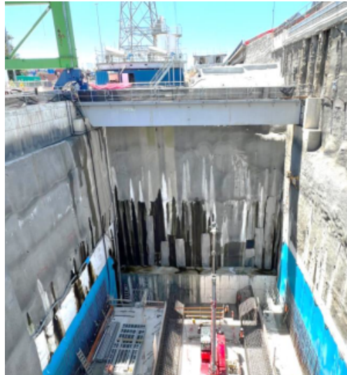
Figure 8: Headwall at southern inbound portal and concrete cradle in the 30m deep retrieval pit
