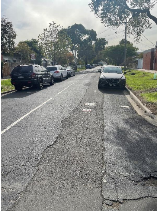
Figure 6 Surface Fittings within Road Reserves
