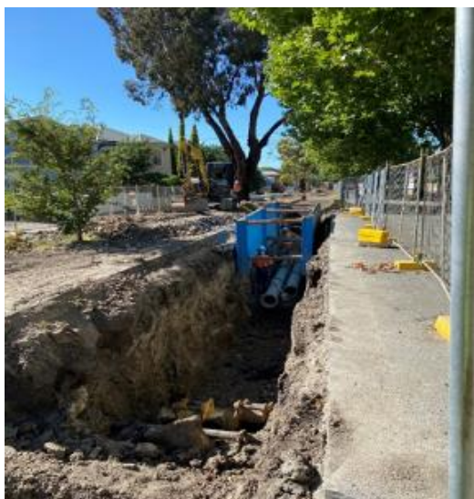
Image: Drainage installation along Melbourne Road from Electra Street end to Pasco Street
