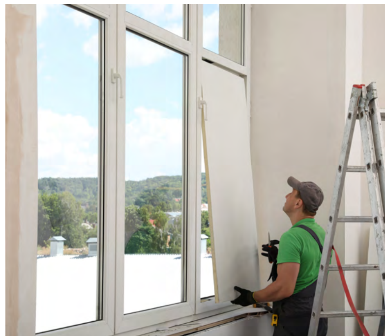
Glazing windows for sound control
