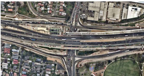
Image: Works at the Williamstown Road interchange showing the Hyde Street ramps and the inbound tunnel portal
