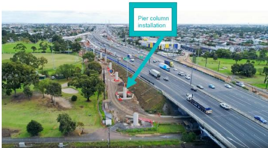
Figure 6: Pier column installation at Donald McLean Reserve as part of the Hyde Street ramp works
