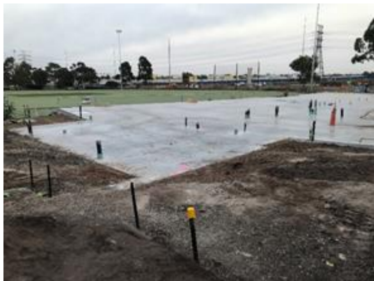
Figure 4: Concrete slab for the new WH Couch Pavilion at Donald McLean Reserve
