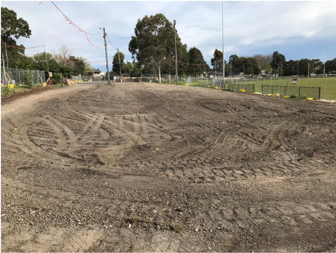
Figure 3: Location of the former WH Couch pavilion at Donald McLean Reserve after demolition
