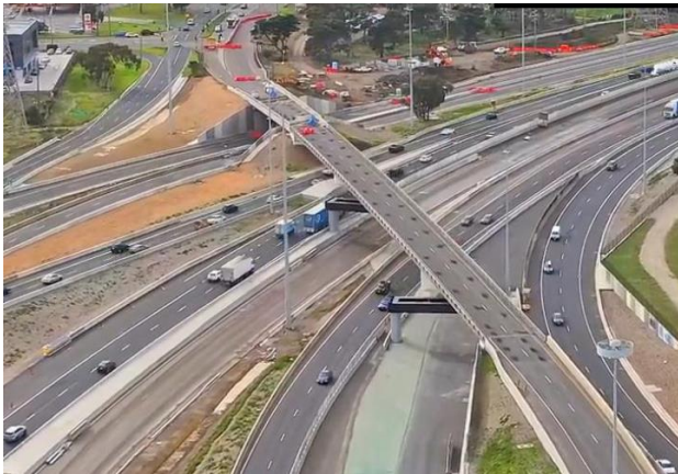
Image: Works at the M80 interchange showing new Geelong Road outbound overpass
