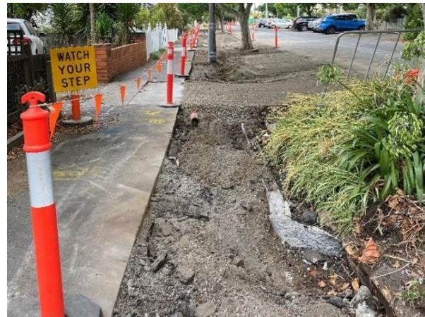
Image: Works along Cecil Street (Thompson Street to Kanowna Street) is also underway with new drainage, kerb and channel being installed
