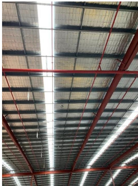
Figure 12 – Internal sprinkler system running throughout the entirety of the warehouse's roof
