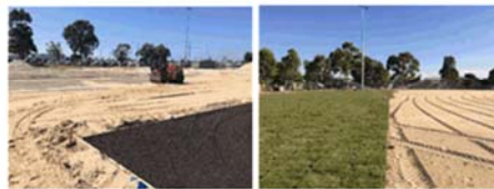
Above: Photos showing the new sand profile, cricket wicket construction and instant turf laying at Bryan Martyn Oval.
