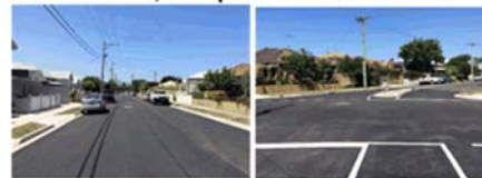
Above: completed works in Alma Terrace, between Bunbury Street to the north of Paine Street intersection is now complete.
